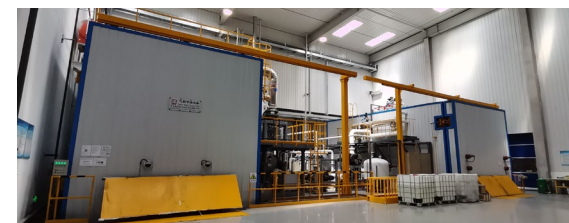
Vapor Phase Drying Plant
